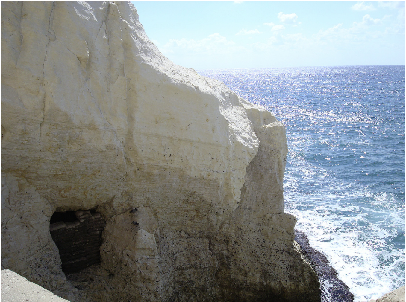
Fig. 12. Blocked tunnel at Rosh Hanikra.
